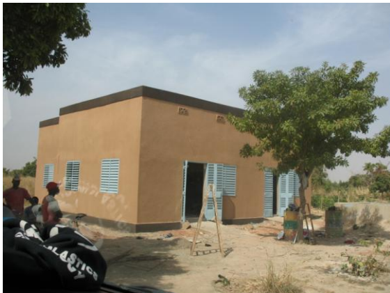
The Dental Clinic is the first building of the Medical Clinic to be built. A foundation has been built for the
